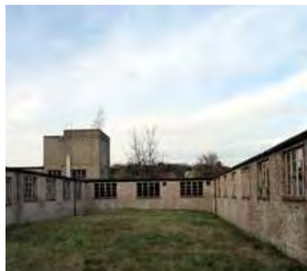
Dilapidated Block G
